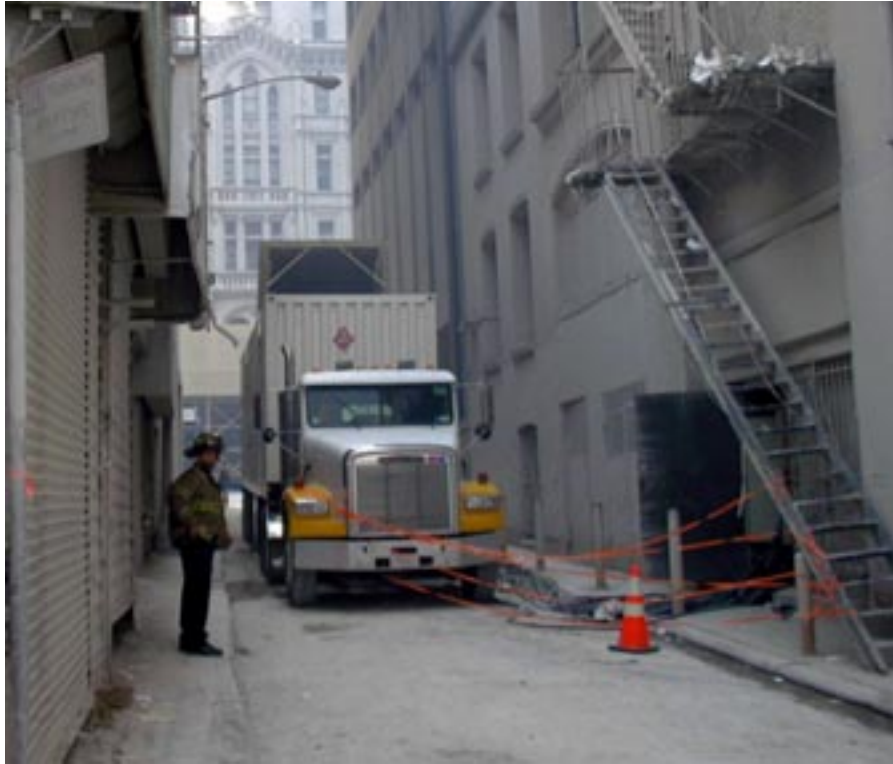
Fig. 2: Portable Diesel-powered Generator
