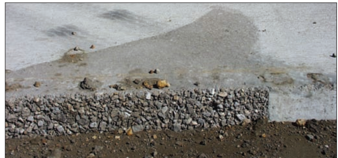
A heavy rain before final set can wash away cement paste and expose course aggregates.
