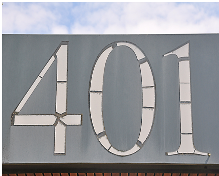
FIG. 2. Cracked lettering at Ecole Polytechnique, Palaiseau, France
