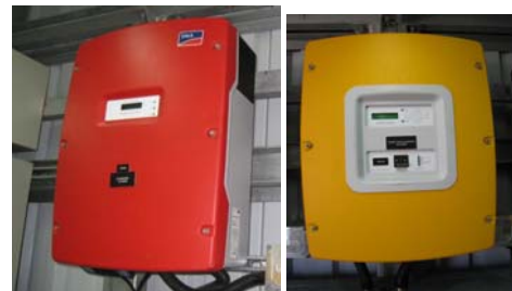
Figure 12-2 The PV Inverter and battery inverter in of the PV System
