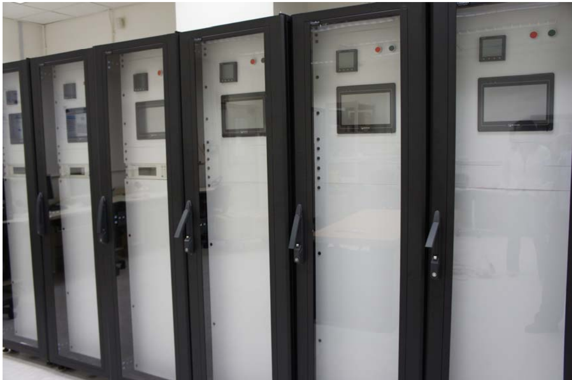
Figure 8-3 Variable-speed CRAC can save up to 40% of fan power consumption.
