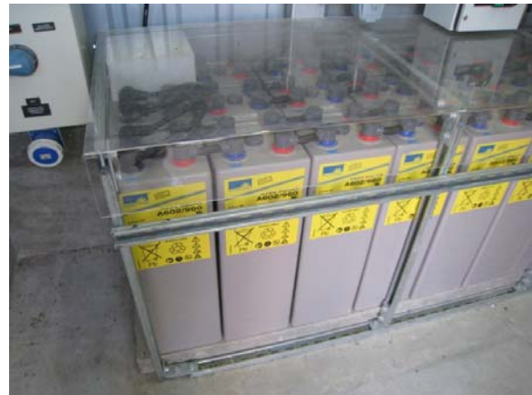
Figure 11-15 Batteries of the Town Island PV System
