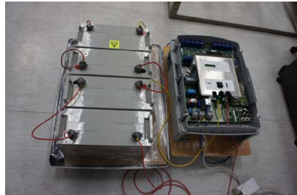
Figure 4-4 Smart meters for battery management
