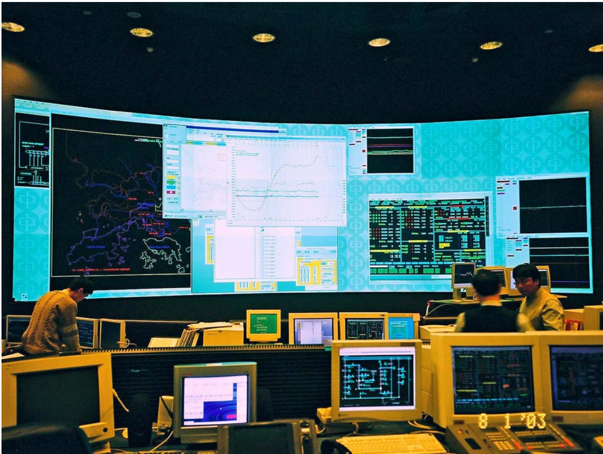
Figure 4-6 The System Control Center of CLP Power
