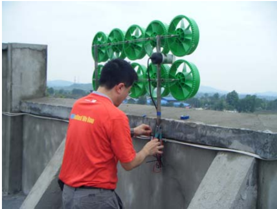
Figure 1-1 The micro wind turbine was installed a reconstructed school in Sichuan.
