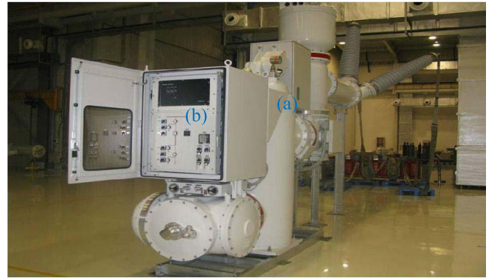
Fig. 2. Example of smart electronics close to HV devices in GIS. (a) HV GIS device. (b) Smart electronics devices.
