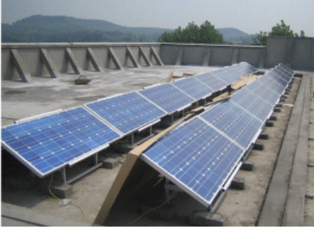
Figure5. Showing the PV array
